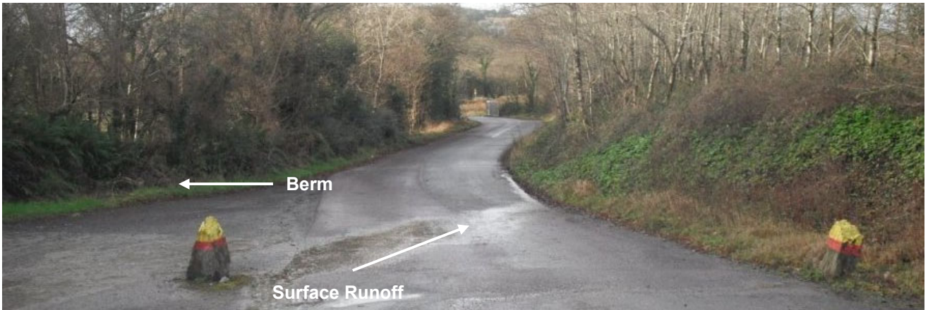
Photo 7.3.23: View West of main access road into the quarry. Note the camber of the road is away from the stream and there is an earthen berm along the road edge almost as far as the access gate.
