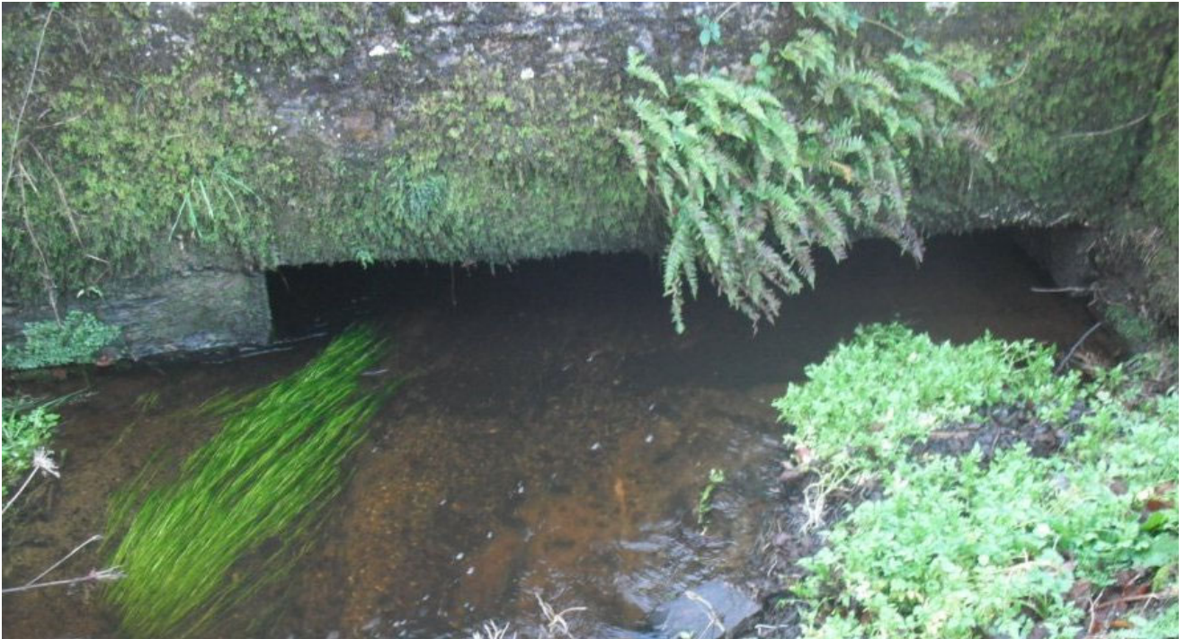
Photo 7.3.28: View of stream flowing under bridge over public road adjacent to access road to quarry. (This is just downstream from where the attenuated quarry stormwater enters the watercourse).
