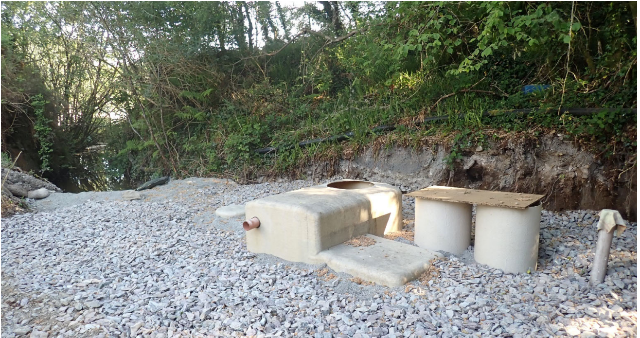
Photo 7.3.15: View of the Pond L overflow with the Tarmac Plant interceptor on discharge Location 04.
