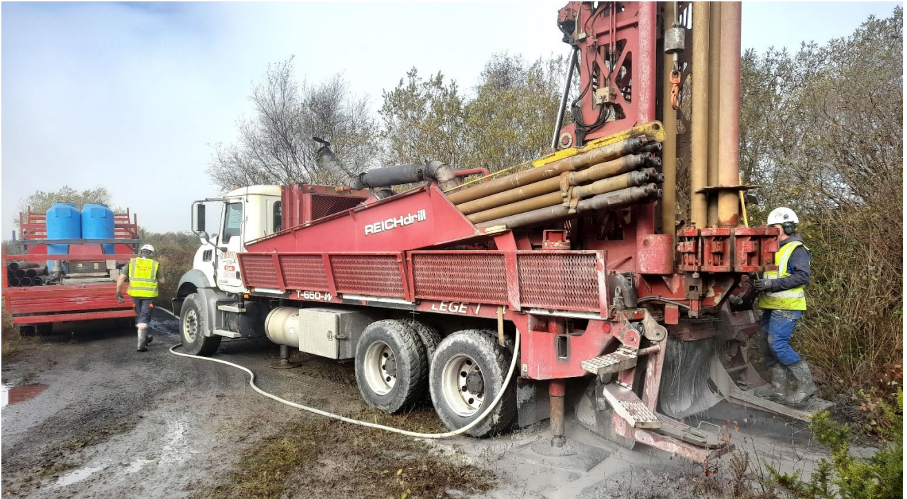
Photo 01: Drilling rig on Location BH03 in the NE area of the site by Pond C. (Tuesday 22 nd Oct 2024).
