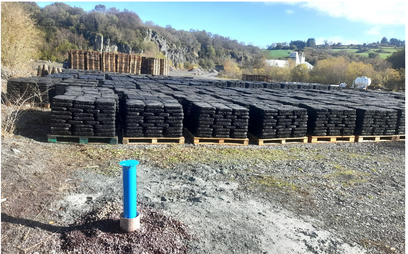
Photo 08: View east of BH02 installed on the upper quarry bench in the Phase 1 expansion area.
