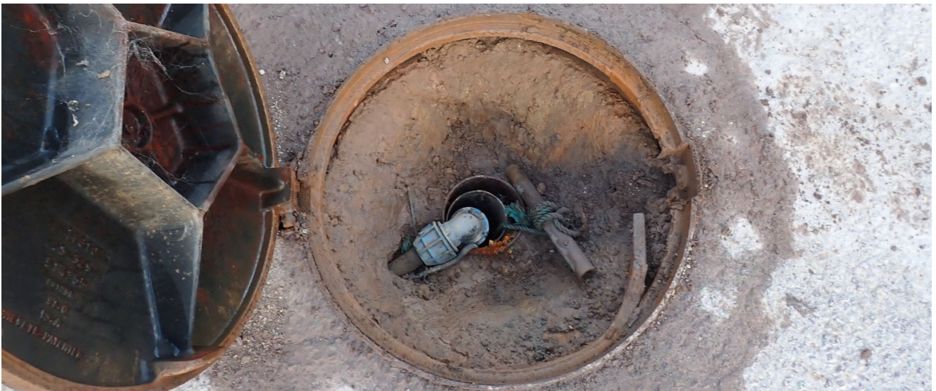
Photo 19: View of Tarmac sites water supply Well headworks.
