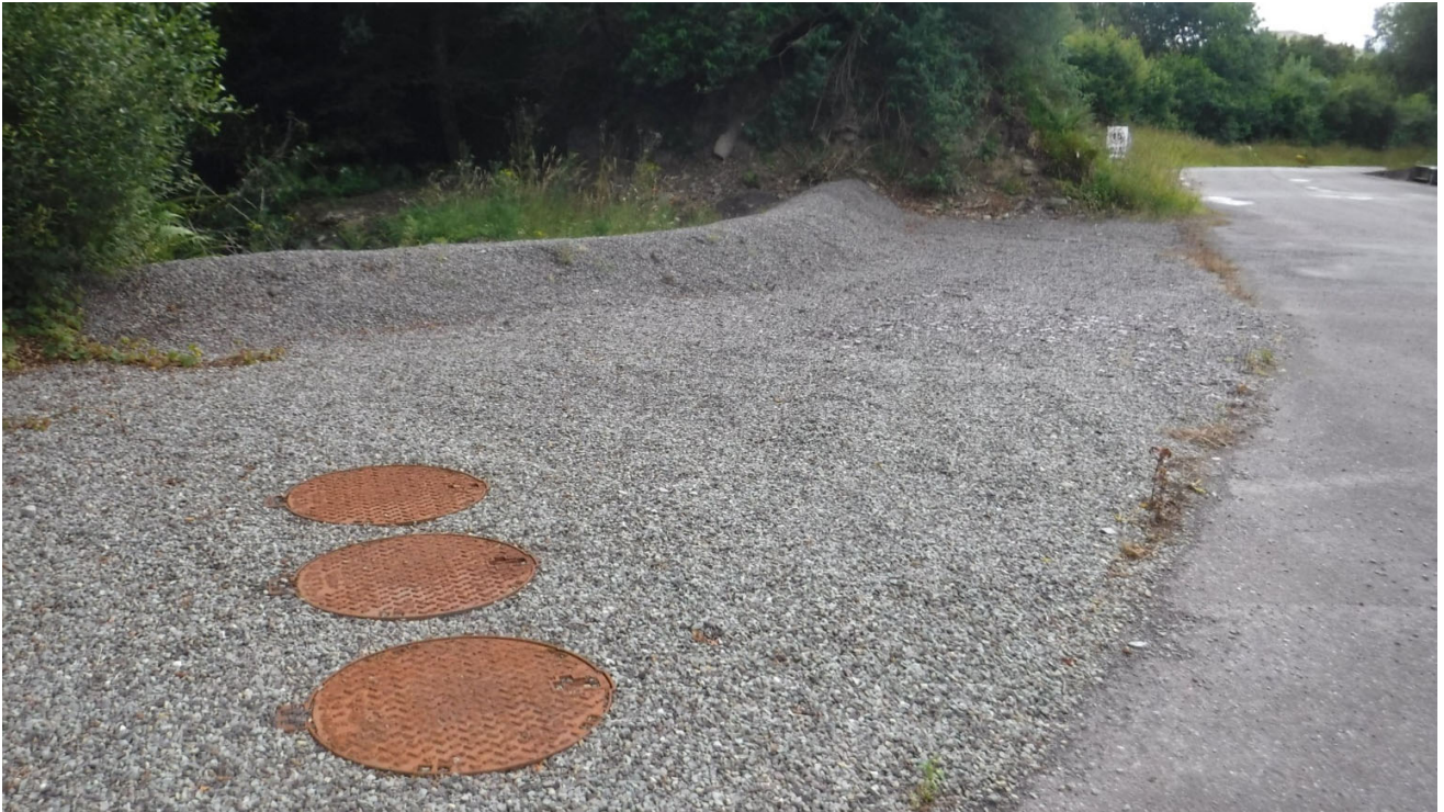
Photo 7.3.10: Manholes of old interceptor on south edge of Tarmac Plant – SW discharge Location 03.
