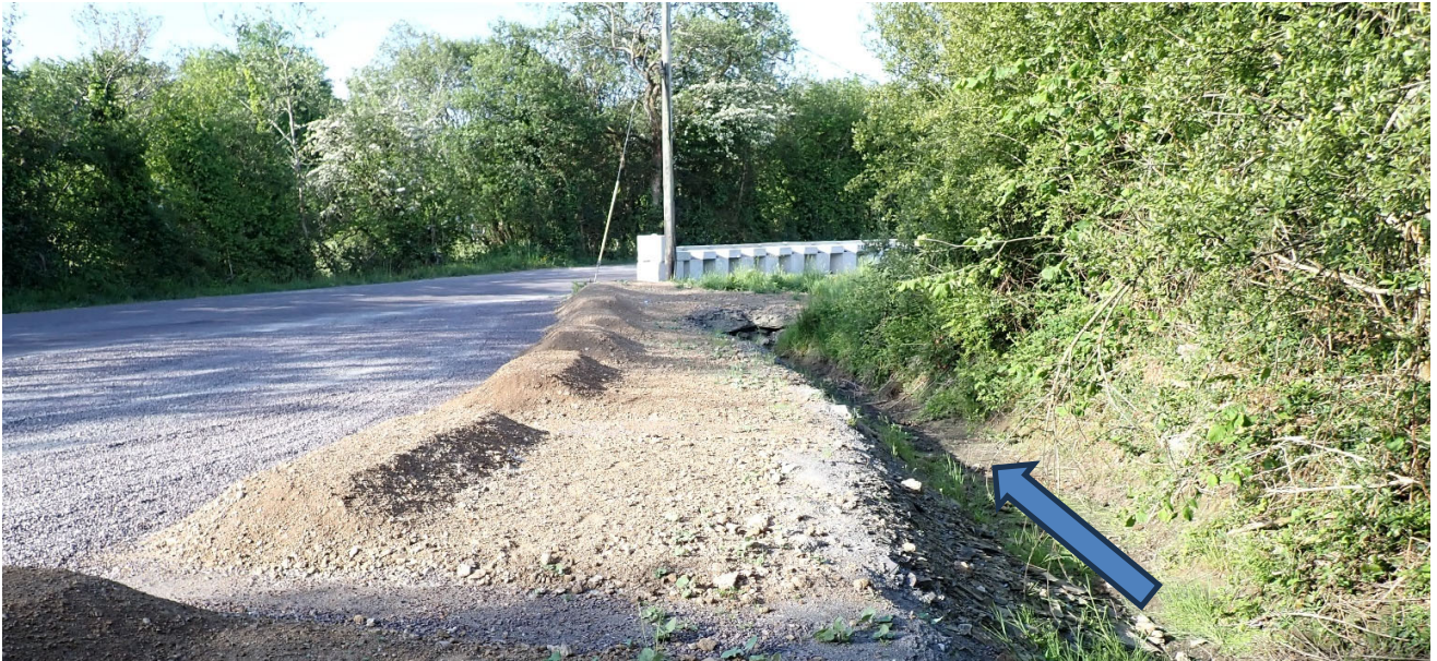
Photo 7.3.21: The sites final outflow drainage ditch going to a pipe under the road and to the stream. This is the Quarry Site Discharge Location 05.
